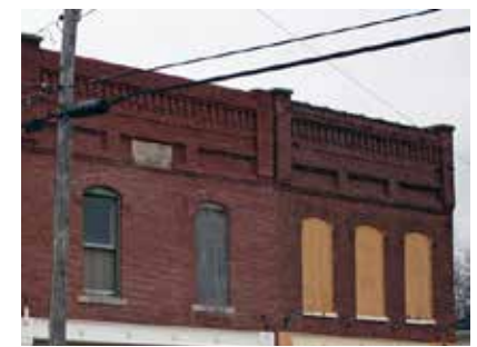
Examples of unrestored and boarded up windows
