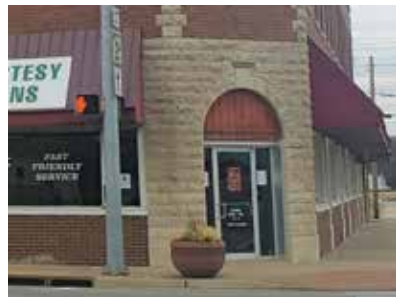
Examples of an inappropriate door with mismatched style and opaque screening
